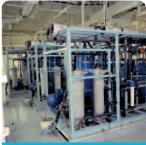
Hatenboer-Water RO system on board Atwood Advantage drillship
